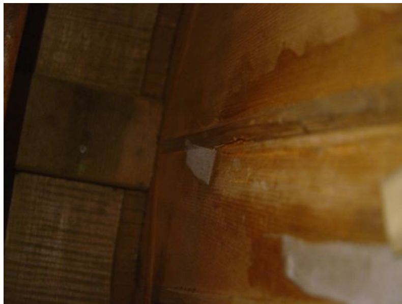
Figure A 22. Interior view of damage on the top and center fan brace (photo courtesy James Westbrook)
