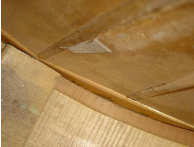
Figure A 21. Interior view of the center fan brace, cloth patch and tail block, focus on the tailblock (photo courtesy James Westbrook)
