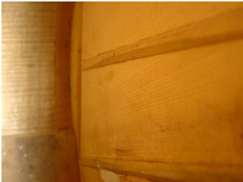
Figure A 18. Interior view of the center fan brace and one treble fan brace (photo courtesy James Westbrook)
