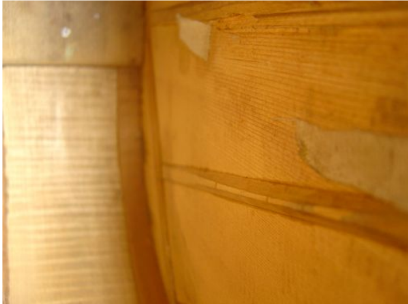
Figure A 19. Interior view of the center fan brace and one bass fan brace (photo courtesy James Westbrook)
